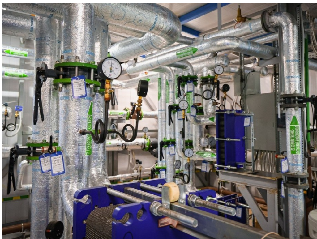
Figure 2. Automated boiler room
